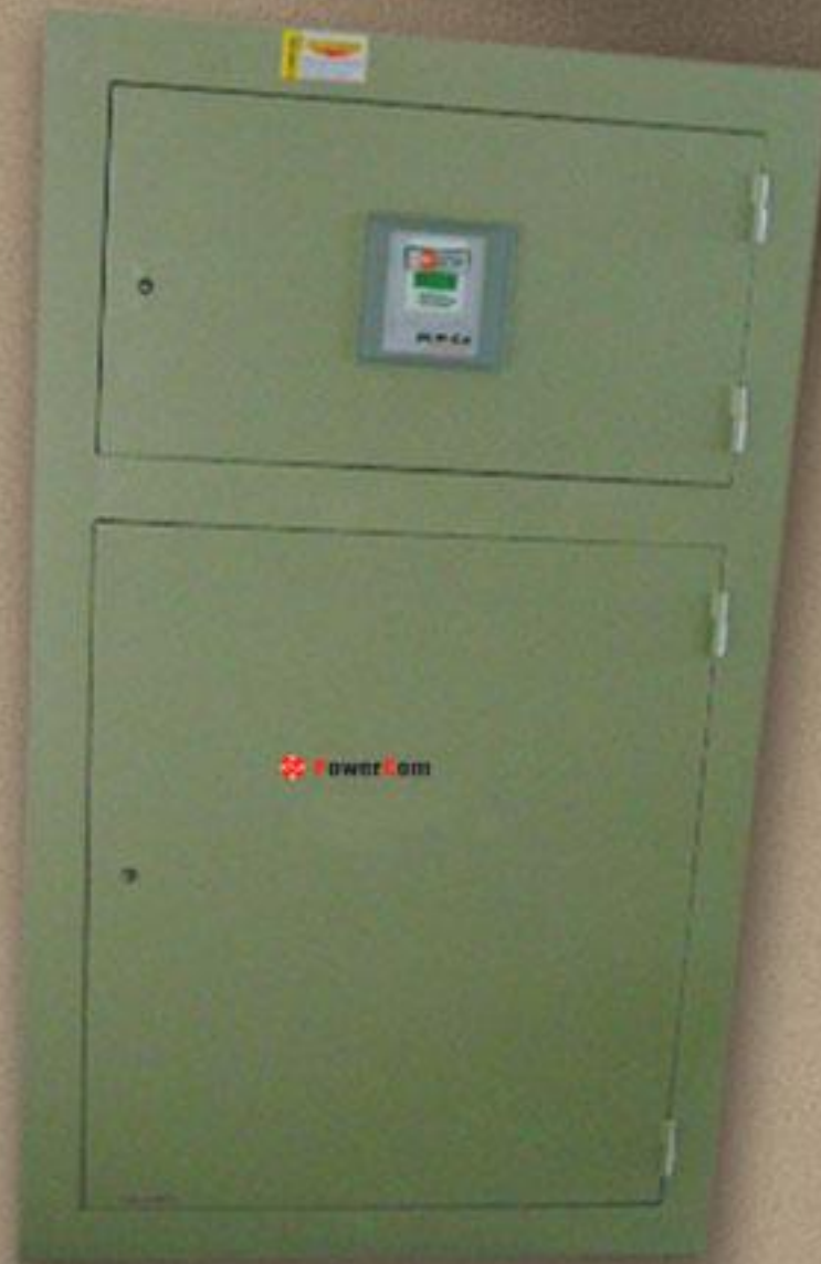
Power Factor Improvement Plant
